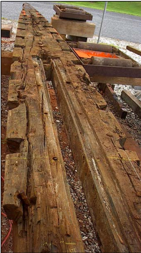
Checks between frame pockets in old oak keel timber
